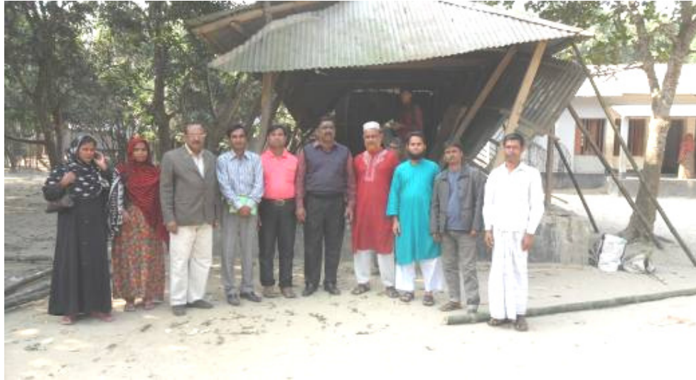
Rubina khatun along with the standing committee members standing in front of damaged shed.
